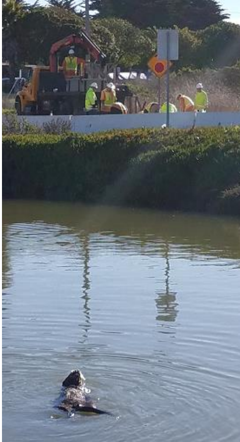
One of the resident sea otters keeps an eye on county work crews during installation of the speed table.
