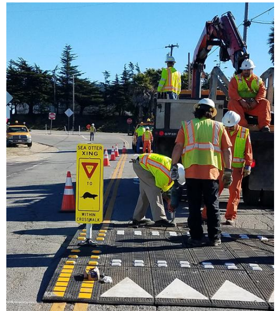
Public Works crews install the speed table on Moss Landing Road (above).
